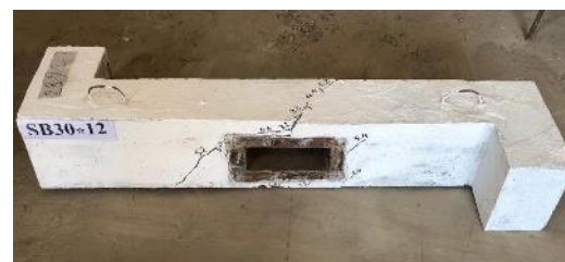
(b) Crack pattern for SB30x12
