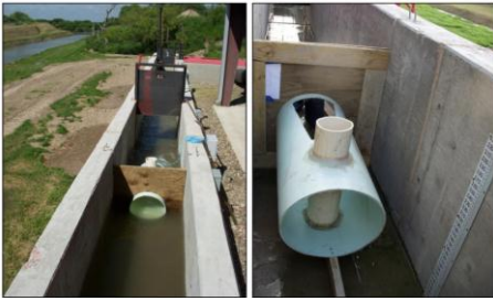
Fig. 2. Calibration of the circular flow meter in the Harlingen Irrigation District.
