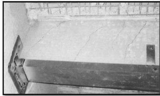
Crack in beam
